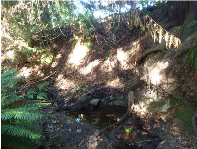
Photo 15. View of 3 m high eroding right bank
